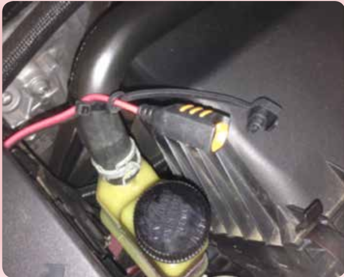
Female connector in my engine bay with the waterproof plug pulled out; the other end of the connector is permanently attached to the battery terminals
